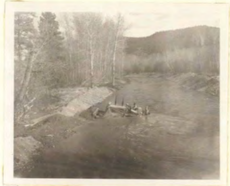
"Seagoing" TD-18 dozer in action. Widening, deepening and straightening channel of Jocko River above No. 1 flood gate.
